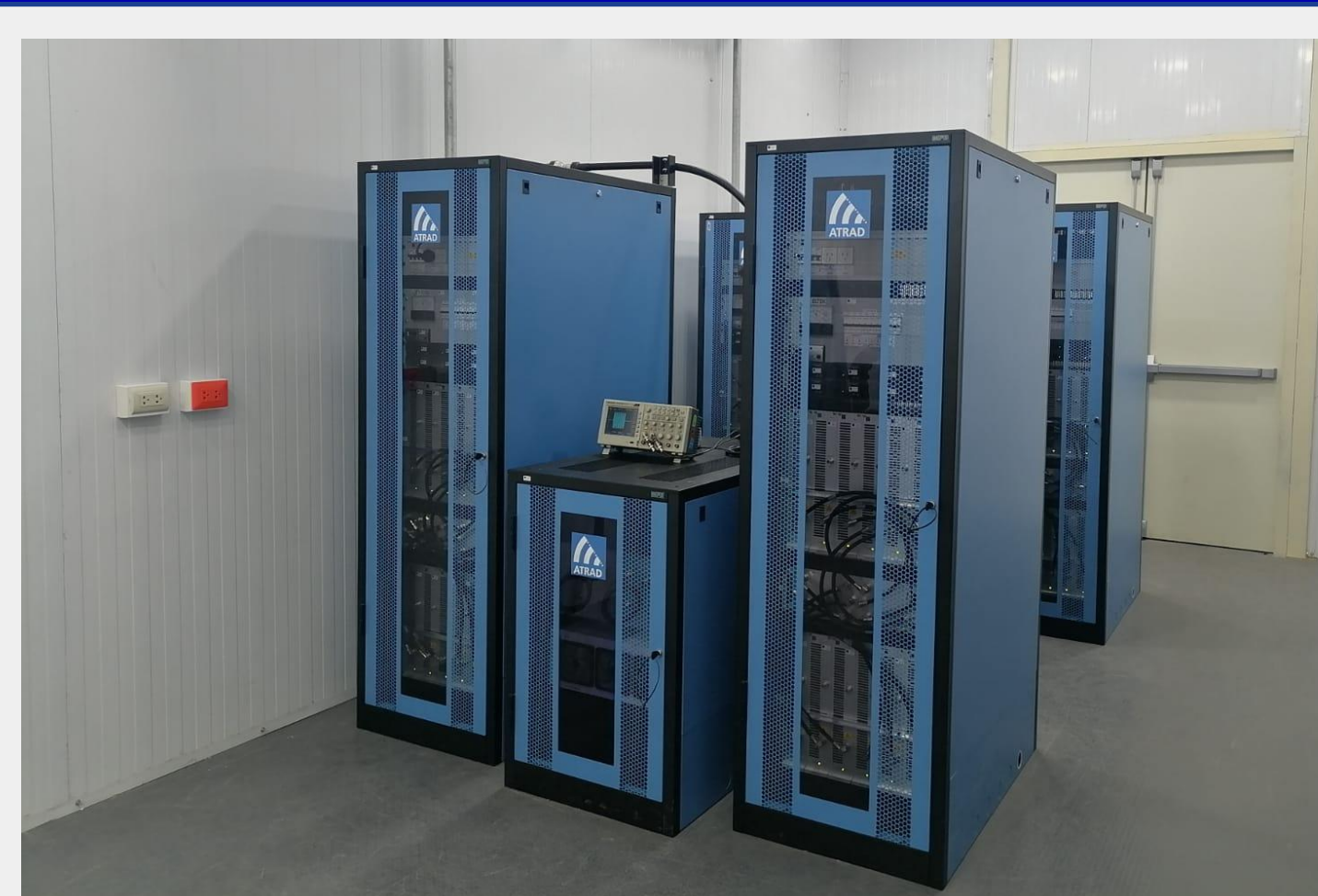
Figure 1. New 96 kw solid-state transmitters
